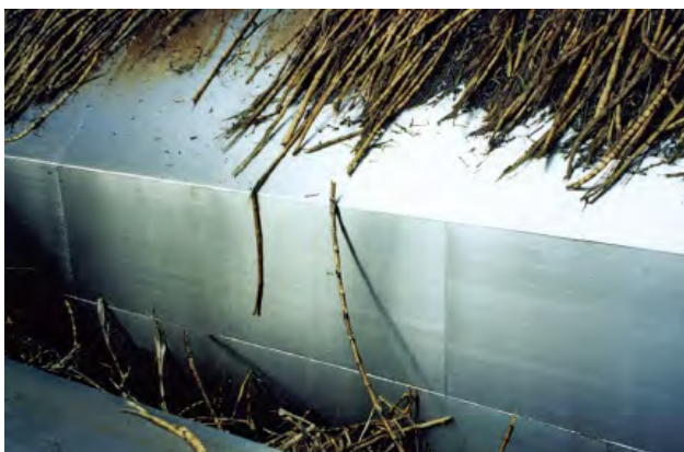
Side of the sugarcane conveyor
